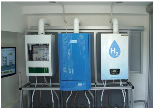
3 pilot hydrogen central heaters
