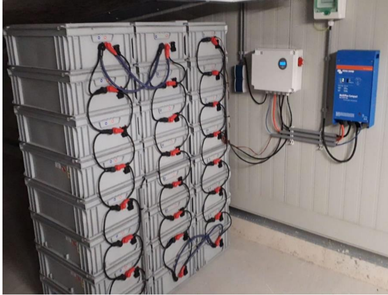
Back up energy storage
