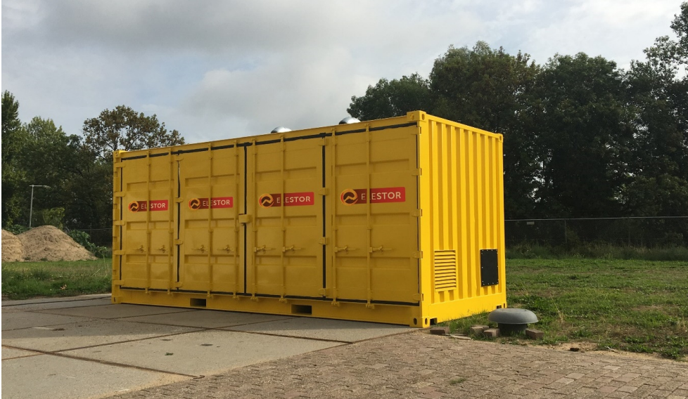
50kW/250kWh HBr Flow Battery system
